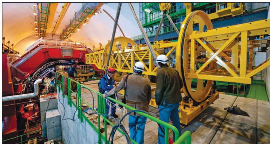
Installation of the EMCal supermodules requires a special insertion device with rails.
